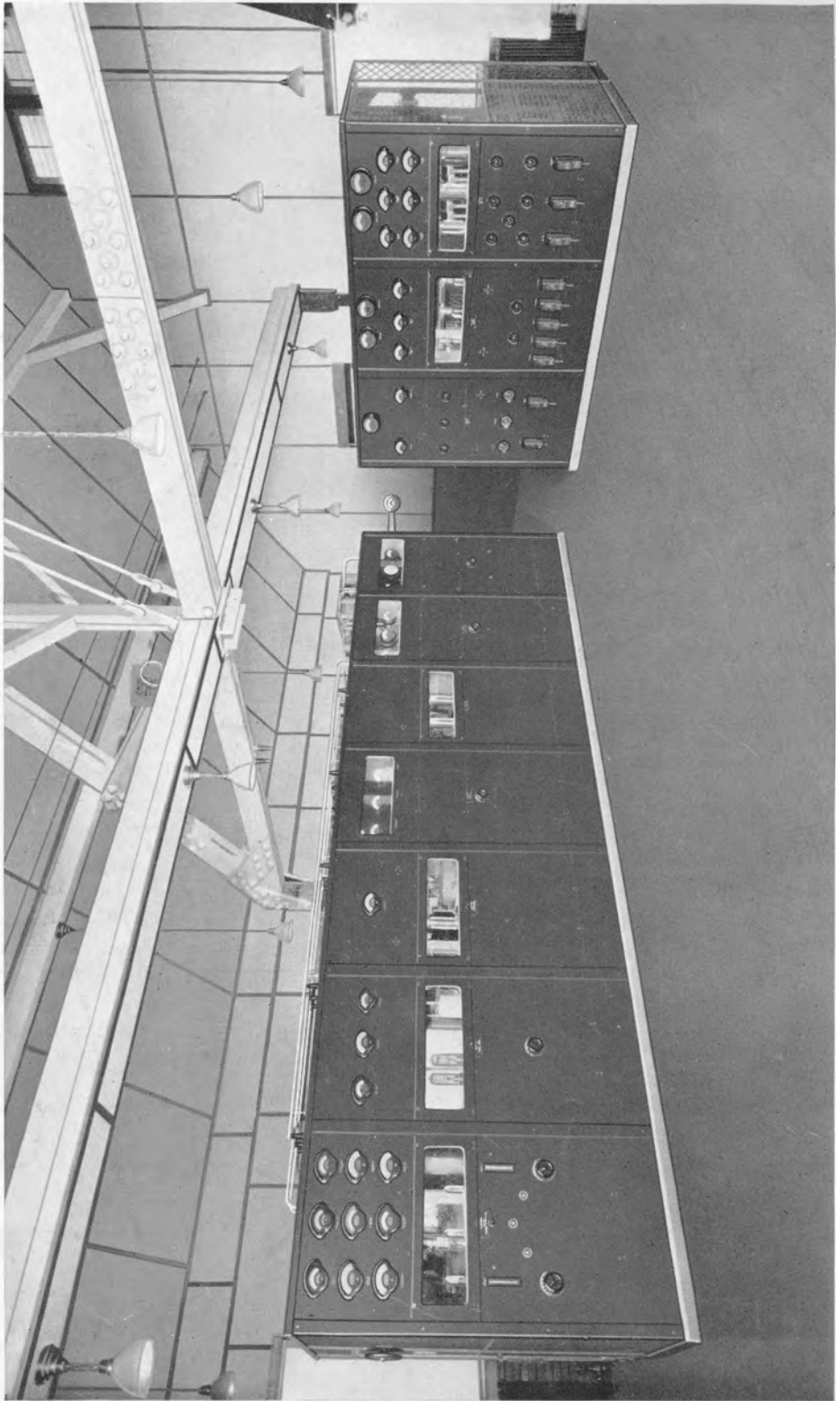
No. 7-A Radio Transmitter
